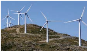
Koudia 100 MW Wind (repowering) Morocco
